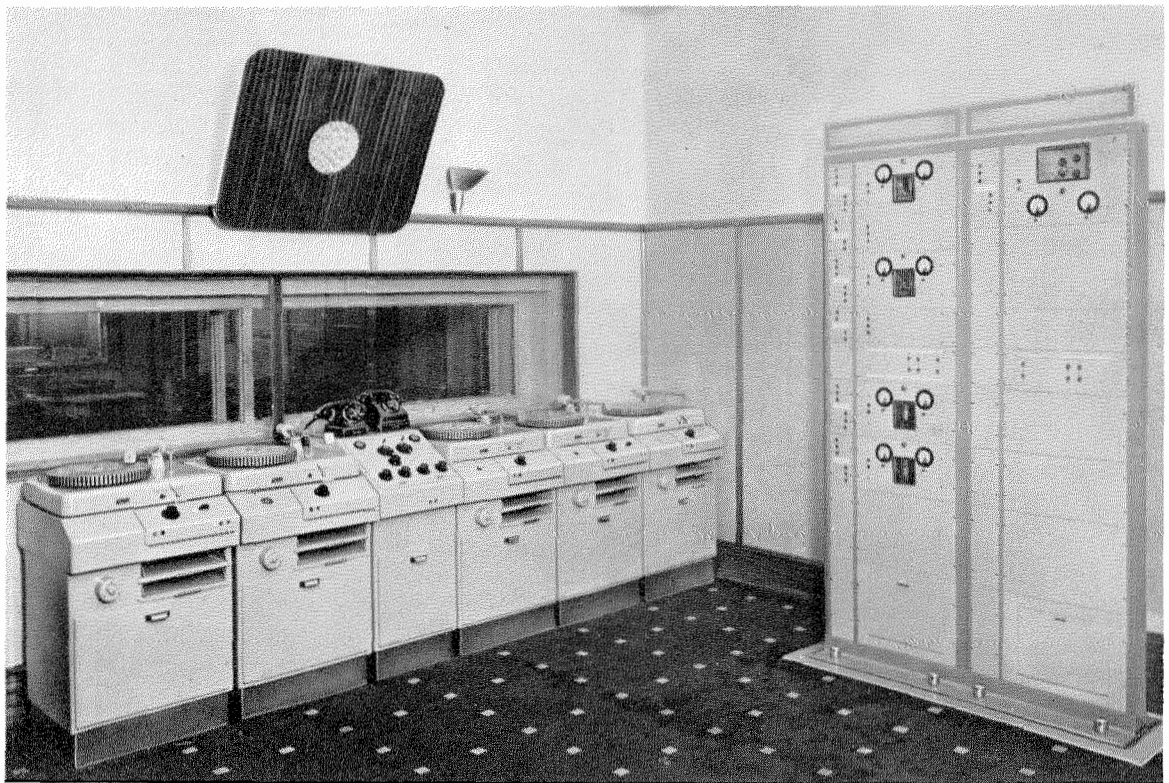
Fig. 3—Turntable desks and equipment racks in an alpha control room.
